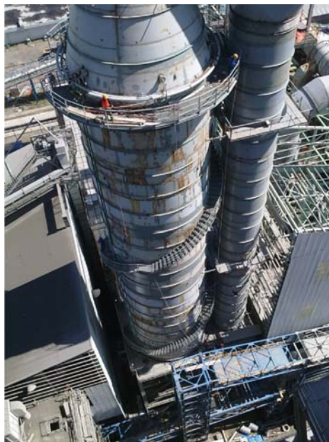
The 95m Gas Cooling Tower at the Lohknga plant to be Scaffolded by AST
